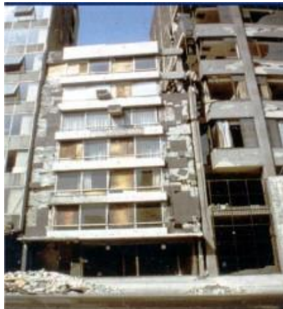
The 1985 Mexico Earthquake (Anagnostopoulos 1988)
